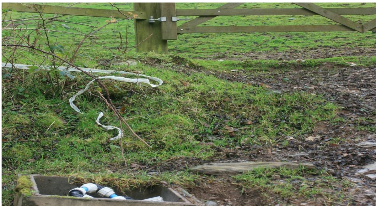
Example of inappropriate arrangements for a borehole. Note the lack of cover and the risk of ingress as the headworks are below the level of the surrounding ground and not protected.
